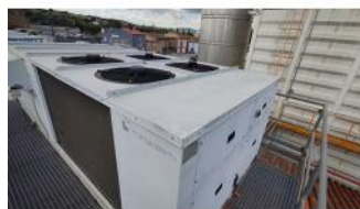
Reference: AGC-009 COOLING UNIT Year: 2006 Brand: CLIMAVENETTA
