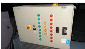
Reference: MOR-244 COOLING UNIT Year: 2001 Brand: C+F
