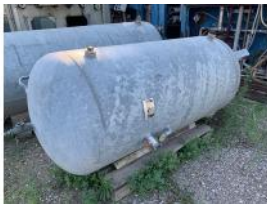
Reference: CCM-028 ACCUMULATION TANK Year: 1992 Brand: X-PAUCHARD
