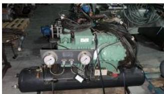
Reference: MOR-197 COOLING UNIT Year: 2009 Brand: TORRECILLA COMP.FRIGORIFICOS
