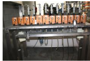
Reference: BPS-066 PUMP GROUP Year: . Brand: PROMINENT
