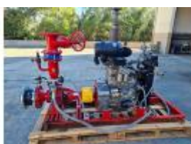
Reference: TES-001 ANTI FIRE EQUIPMENT Year: 2006 Brand: MWM Motores Diesel LTDA
