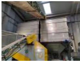
Reference: MZA-007 STORAGE HOPPER Year: 2018 Brand: .
