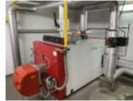
Reference: LFR-113 HOT WATER BOILER Year: . Brand: ROCA
