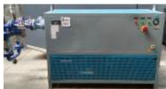
Reference: FTR-023 COMPRESSED AIR DRYER Year: . Brand: ABC
