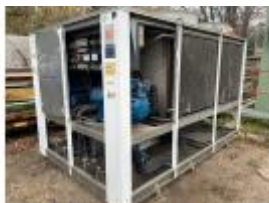
Reference: SLL-010 WATER CHILLER Year: 2001 Brand: HITSA
