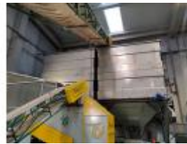
Reference: MZA-008 STORAGE HOPPER Year: 2018 Brand: .
