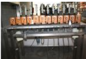
Reference: BPS-066 PUMP GROUP Year: . Brand: PROMINENT
