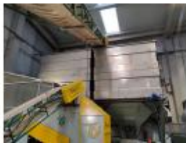
Reference: MZA-008 STORAGE HOPPER Year: 2018 Brand: .
