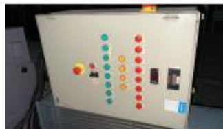
Reference: MOR-244 COOLING UNIT Year: 2001 Brand: C+F
