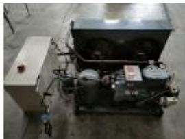
Reference: MOR-241 COOLING UNIT Year: 2001 Brand: .
