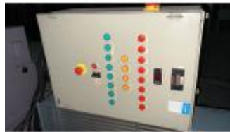
Reference: MOR-244 COOLING UNIT Year: 2001 Brand: C+F
