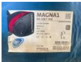
Reference: LFR-098 BOOSTER PUMP Year: . Brand: GRUNDFOS
