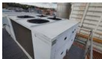
Reference: AGC-009 COOLING UNIT Year: 2006 Brand: CLIMAVENETTA
