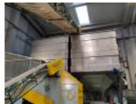
Reference: MZA-007 STORAGE HOPPER Year: 2018 Brand: .
