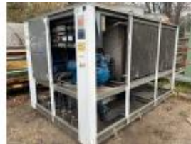
Reference: SLL-010 WATER CHILLER Year: 2001 Brand: HITSA
