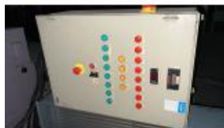
Reference: MOR-244 COOLING UNIT Year: 2001 Brand: C+F
