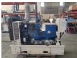
Reference: CCM-040 GENERATOR SET Year: 2001 Brand: FG WILSON
