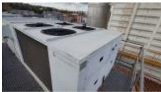
Reference: AGC-009 COOLING UNIT Year: 2006 Brand: CLIMAVENETTA
