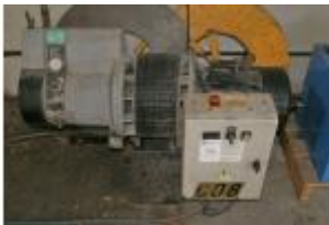
Reference: JHA-031 AIR COMPRESSOR Year: . Brand: COMP AIR
