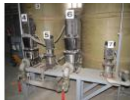
Reference: SER-083 PUMPS Year: . Brand: .
