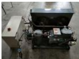
Reference: MOR-241 COOLING UNIT Year: 2001 Brand: .
