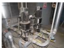
Reference: SER-084 PUMPS Year: . Brand: .
