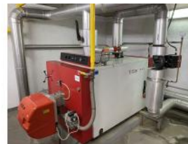
Reference: LFR-113 HOT WATER BOILER Year: . Brand: ROCA
