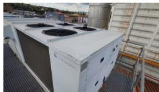
Reference: AGC-009 COOLING UNIT Year: 2006 Brand: CLIMAVENETTA
