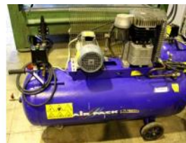
Reference: TPL-020 COMPRESSOR Year: 1997 Brand: AIR PACK
